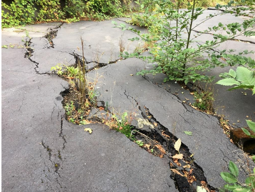
Figure 13. Transverse crack extending through flexible pavement surface.
