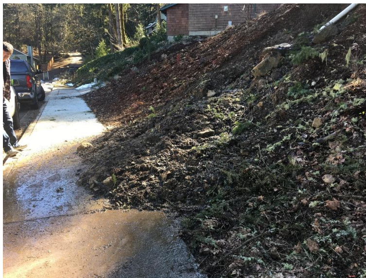
Figure 15. Slope failure due to excess ground moisture.
