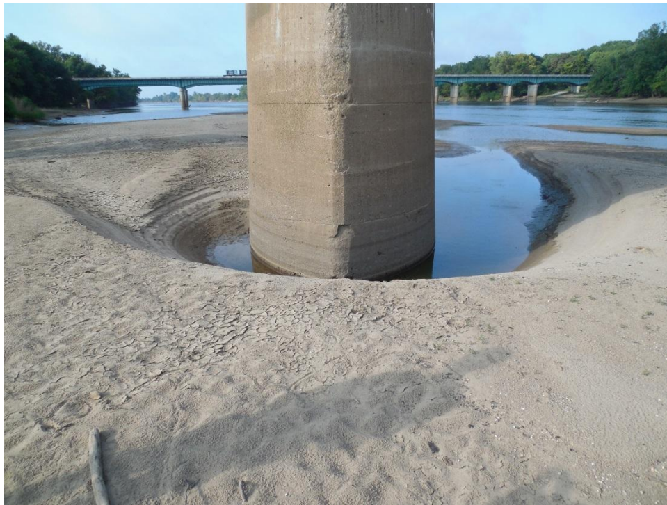
Figure 28. Scour around bridge pier (courtesy of USGS ).
