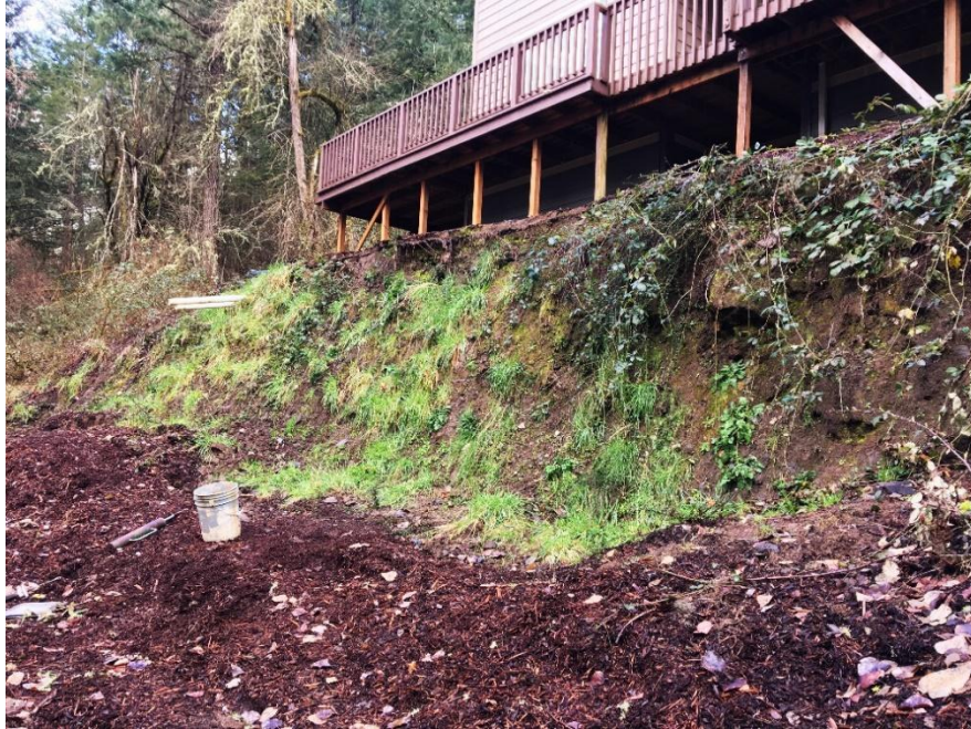
Figure 12. Deep scarps forming behind residential construction.
