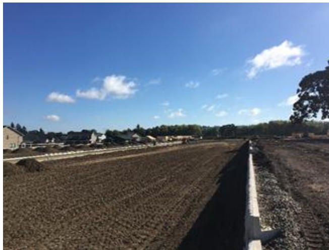
Figure 31. Roughened surface after soil compaction.
