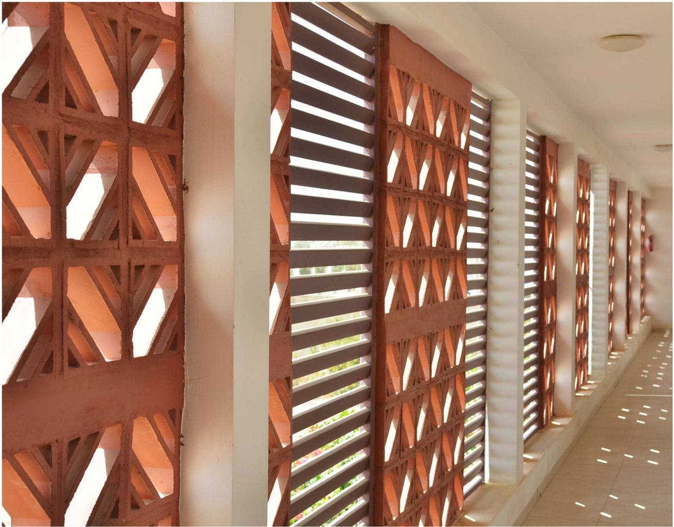
Fig 02. - Overlooking a central garden courtyard, locally-sourced clay ventilation blocks provide sun-shading and passive cooling for interior spaces within SIL's Bible Translation Center, designed by EMI in Senegal (Photo by Matthew Coffey)
